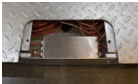
Internal view junction box Galvanized base
