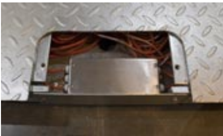
Internal view junction box Galvanized base
